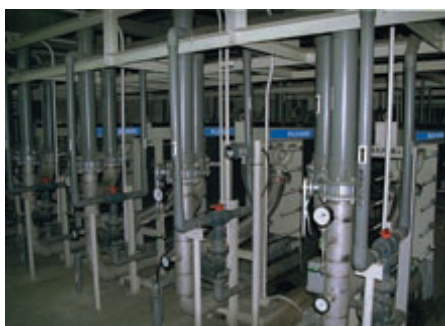
Fig. 9. Pleiade® MBR membrane bioreactor for treating 1000 m 3 /day of effluent from www.vic-ws.it/site/down/PLEENG0411.pdf
